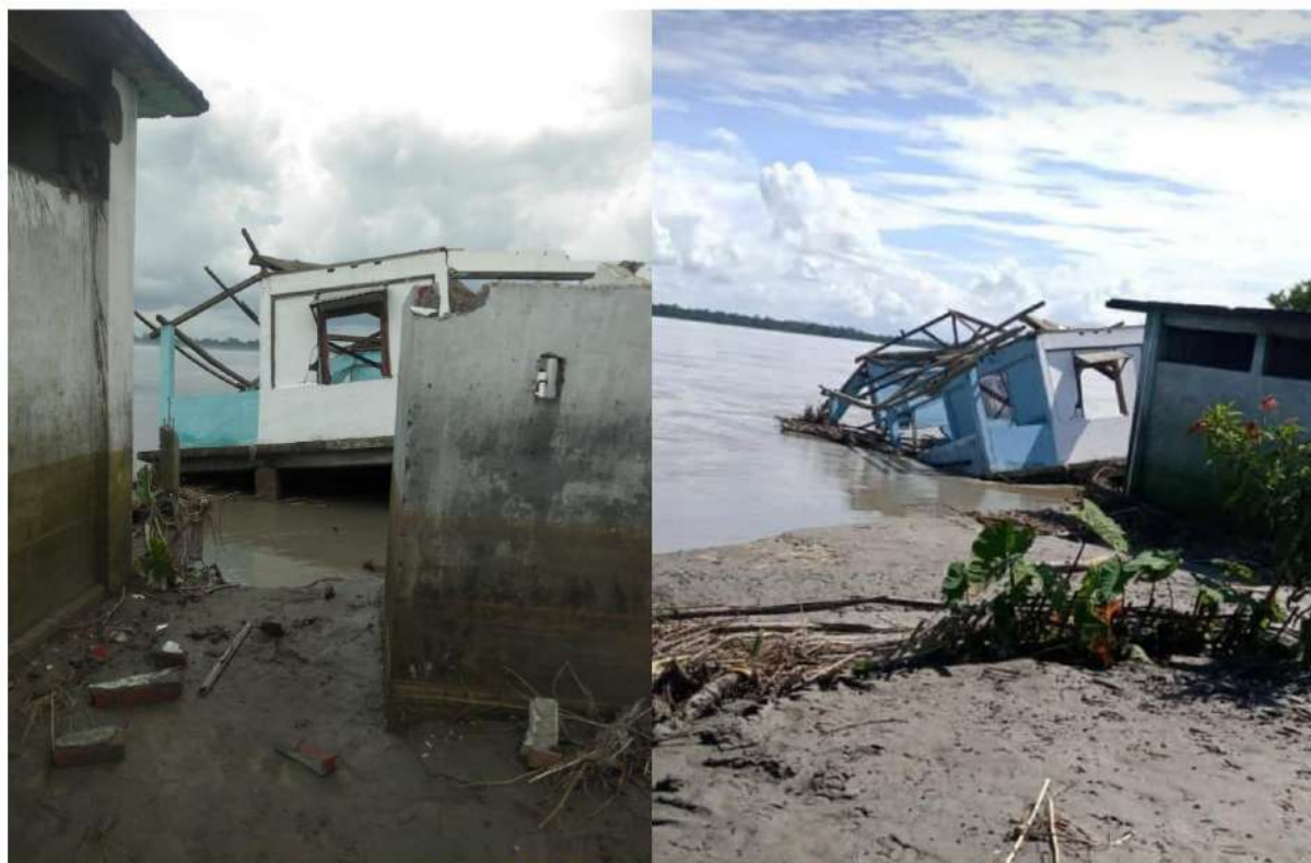
Picture-2 & 3: The images of the broken house
